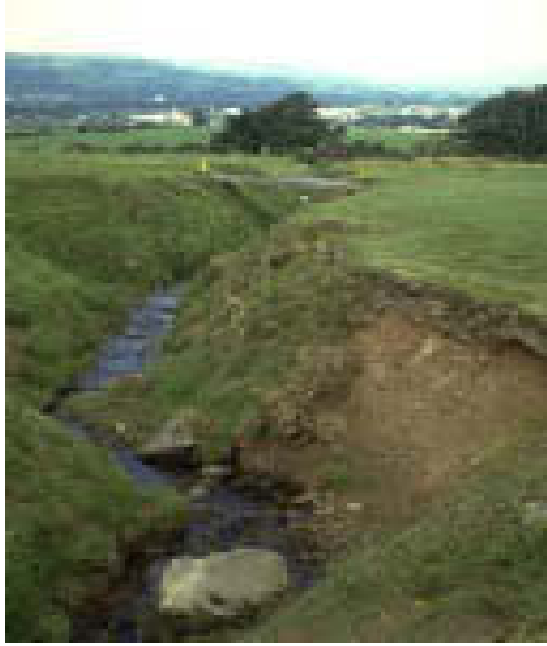
Figure 7 Stream bank instability at Vale of Leven
