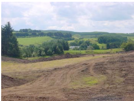
Golf course construction in the wider landscape context: new holes under construction at Eastwood Golf Club, Renfrewshire
